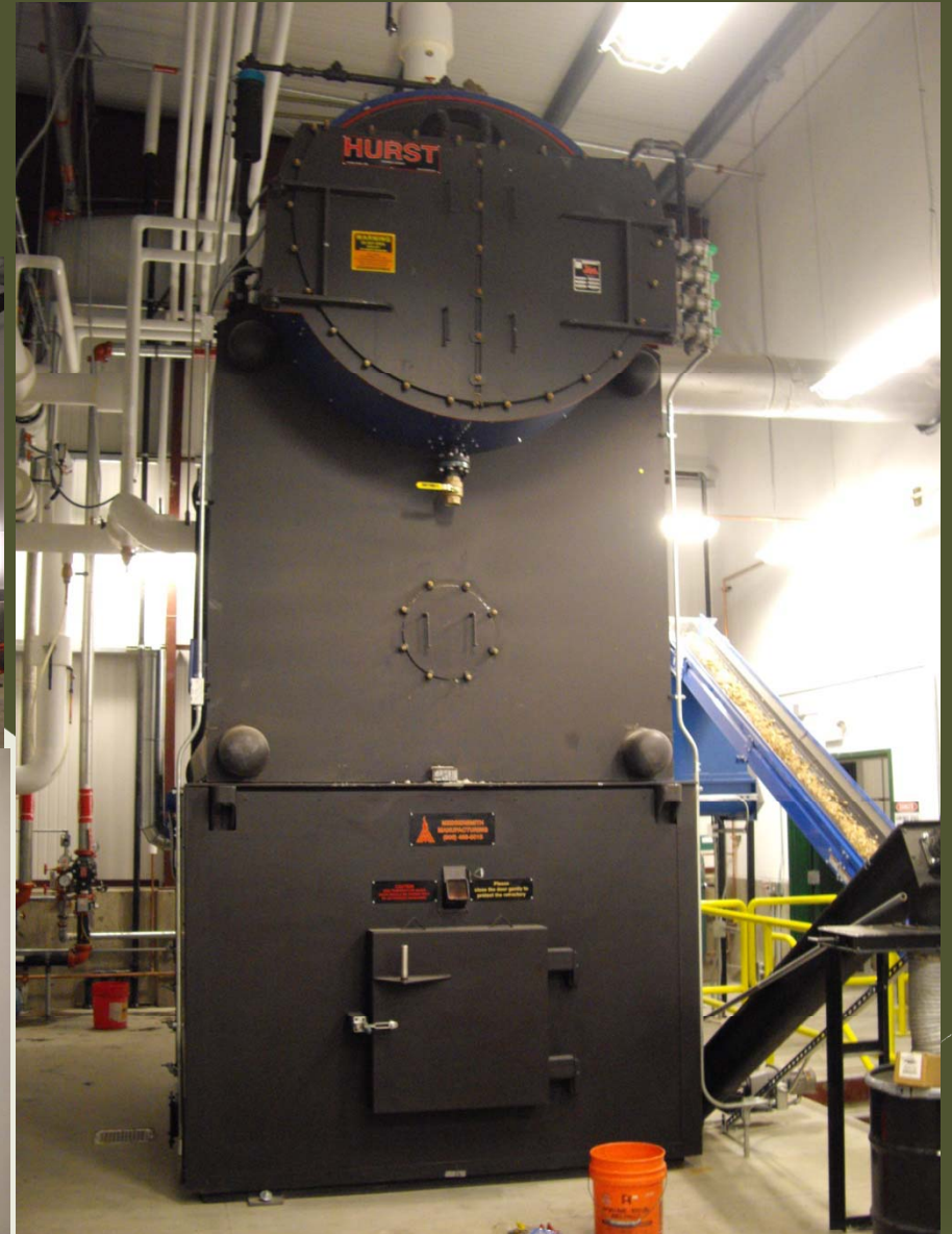
Tok School Wood-Fired Boiler
